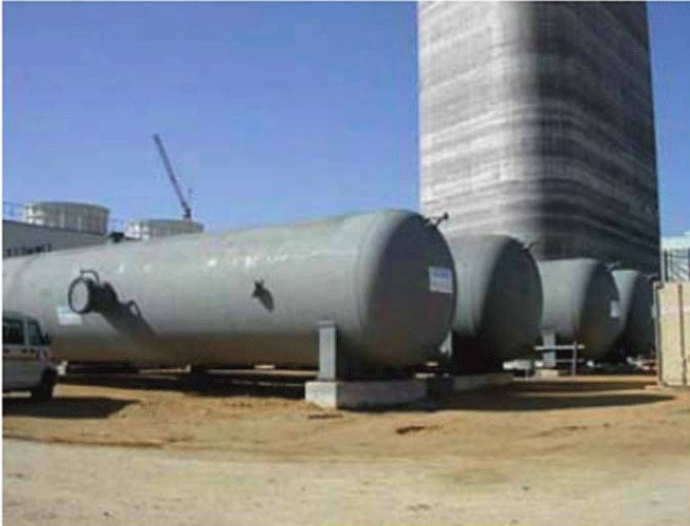
Storage tanks at the PS10 facility ABENGOA
