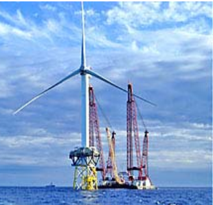
5 MW RePower Beatrice Project
